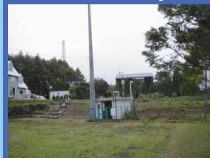
大気測定局 Air Pollution Monitoring Station
